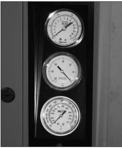
Discharge pressure, filter restriction, and temperature gauges.
